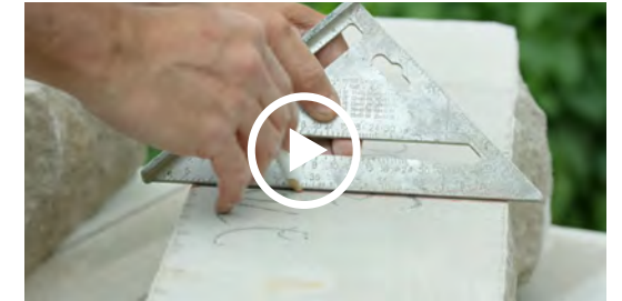
HOW TO BUILD A DRY-STACK LOOK STONE WALL USING POLYCOR GARDEN WALL PRODUCTS
