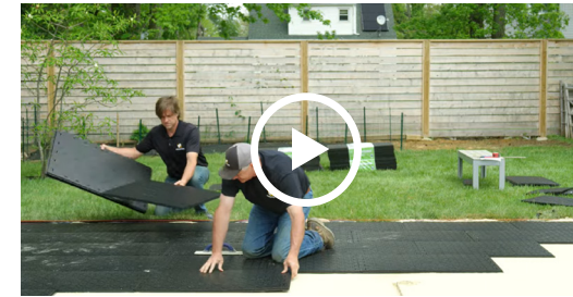
HOW TO INSTALL A GRANITE SLAB PAVER PATIO IN HALF THE TIME WITH EZ BASE
